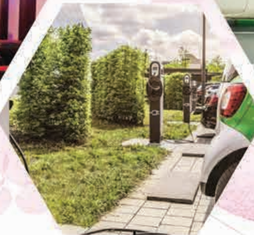
EV CHARGING POINT
